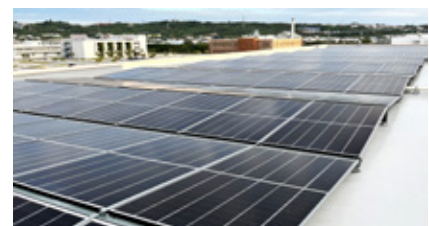
Solar panels installed on the roof of IT Shinryo Park Corporate Cluster Building No. 7
